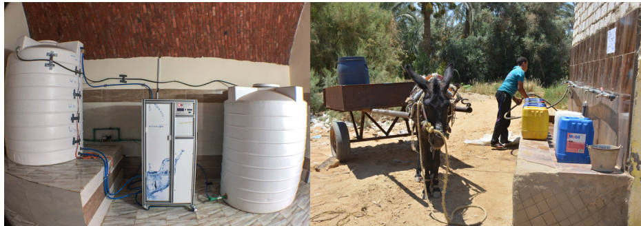
Fig. 8 Water purification system working on solar energy and using anodic oxidation for drinking water purification installed in Egypt's Western Desert (picture source: Kohler for AUC, 2018; authors, 2016).
