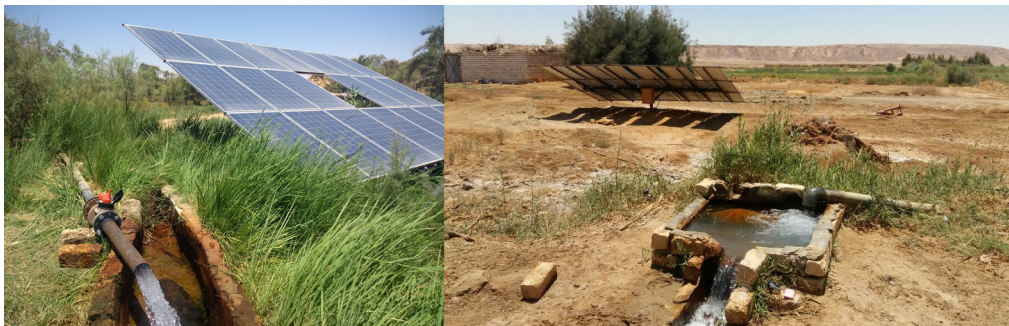
Fig. 6 Examples of solar PV pumps installed in the oasis of El Heiz, in Egypt’s Western Desert (source: authors).
